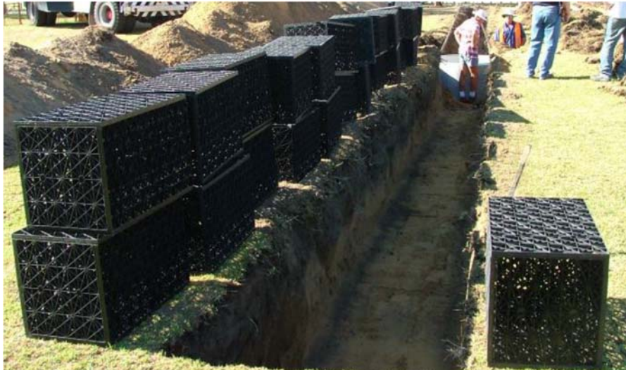
Figure 5 Construction of infiltration galleries using Atlantis Flo-Tank® modules at Floreat in 2008 (Toze and Bekele 2009).
