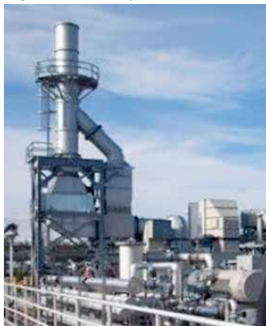
Figure 10 EBMUD's gas turbine cogeneration facility 32 .
