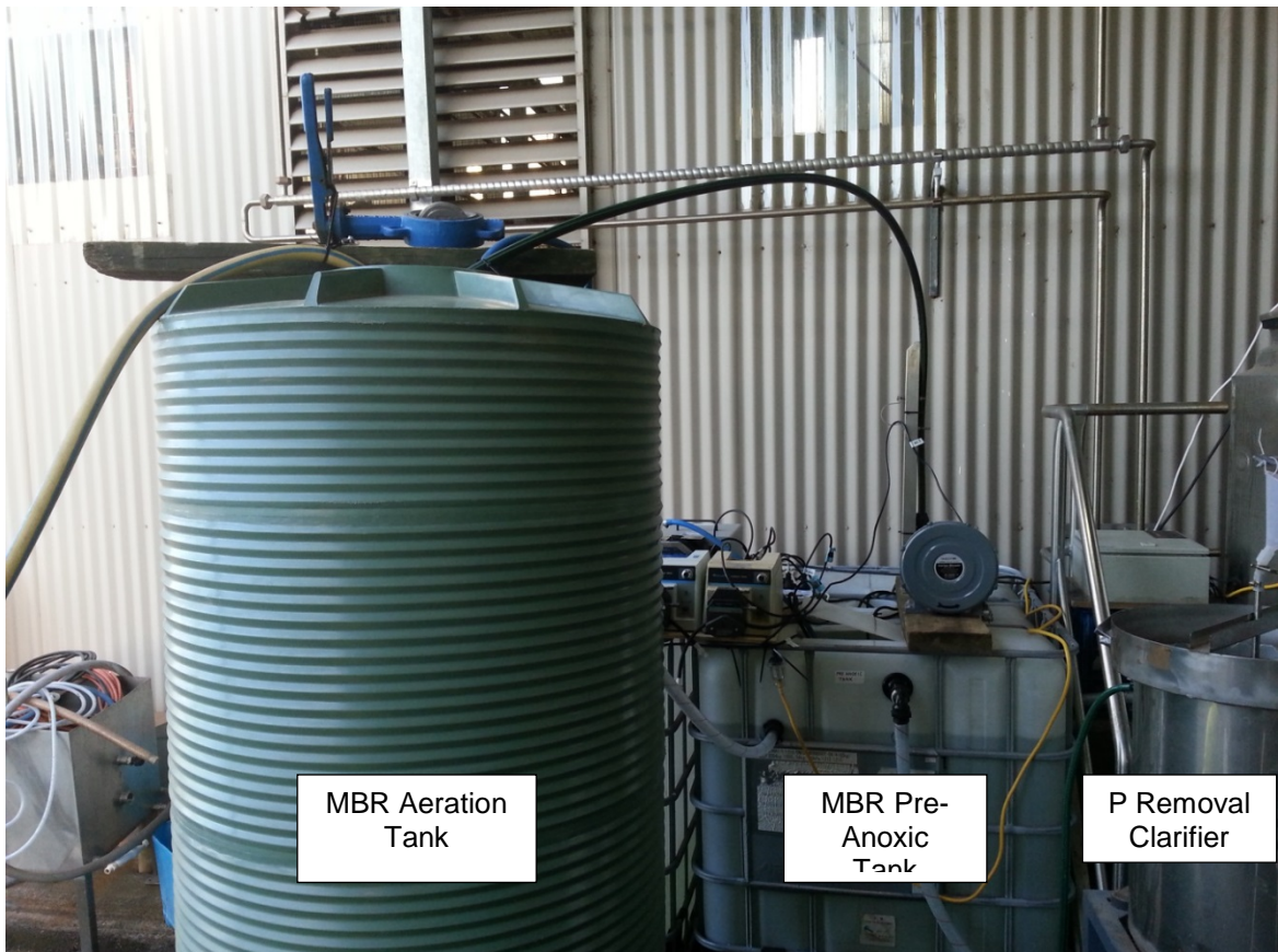
Figure 13. MBR system pre-anoxic and aeration tanks, with the clarifier from the phosphorus removal system in the foreground.
