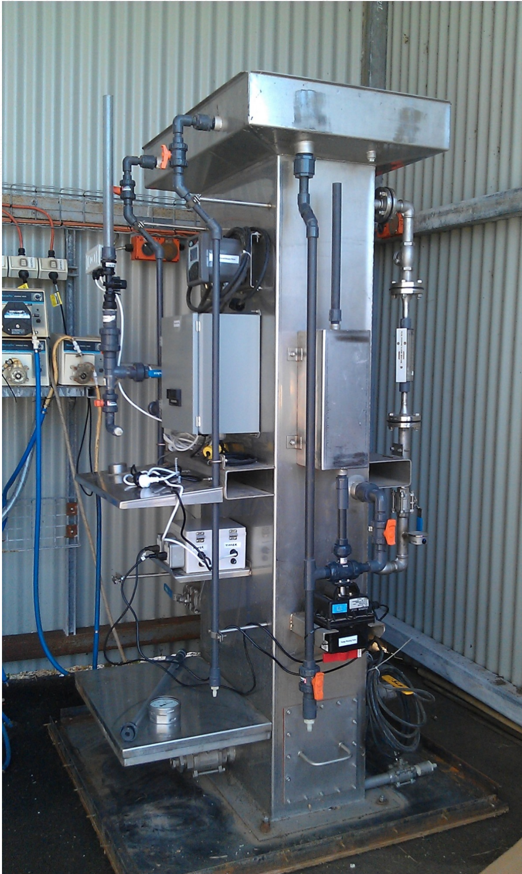
Figure 14. MBR system aerobic membrane tank.
