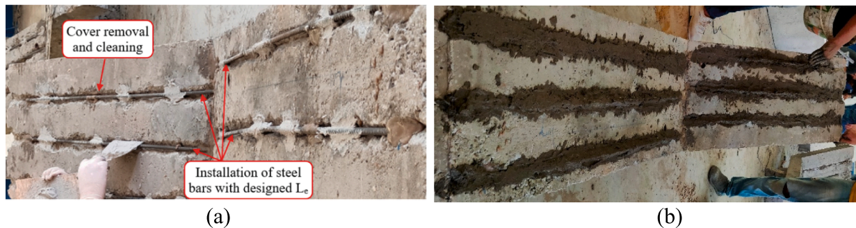
Fig. 8. Strengthening preparation using NSMSB for Group G2: (a) surface adapting and installation of steel bars; (b) re-covering of concrete surface by ECC.
