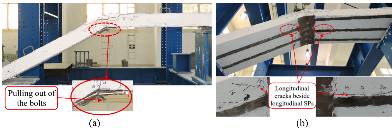
Fig. 10. Crack patterns of slab S-E-LSPs: (a) pulling out of the bolts; (b) cracks parallel to longitudinal steel bars.
