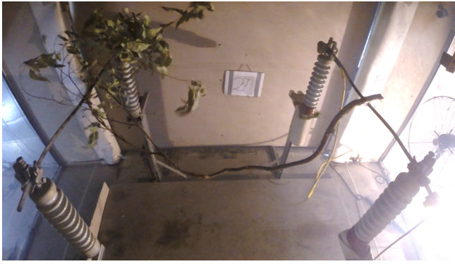
Fig. 15. The branch at 24 s into the recording. The branch is yet to experience any charring, any breakout of flames, and no embers are being shed (VT271).
