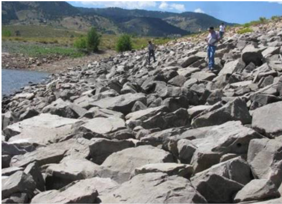
Figure 2.7: Rip Rap with 60 years of history, Horsetooth Dam (Source: USBR, 2012)
