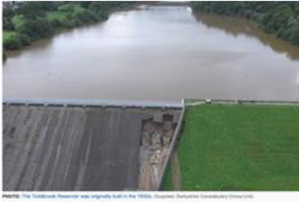
Figure A.7: Toddbrook Reservoir (Source: damfailures.com, 2020)
