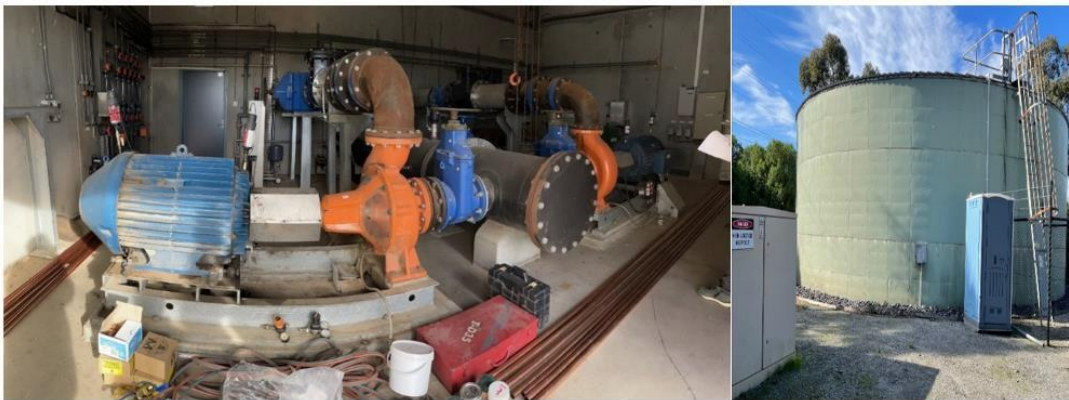
Figure 3.4: Panoramic Photo of the Loemans Road Pump Station (Left) and Shepherds Lane tank (Right)
